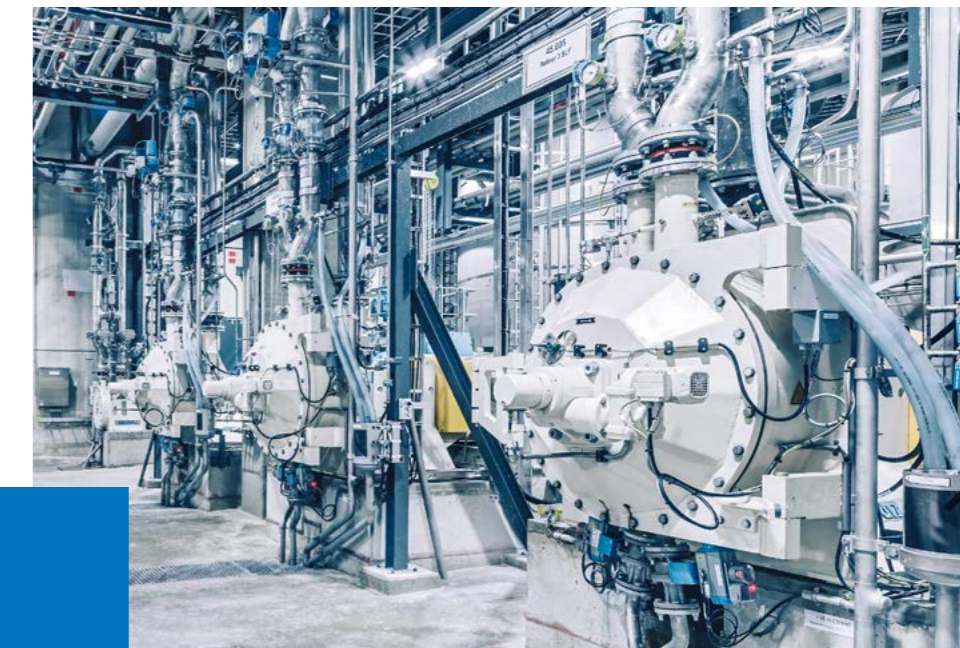
Five TwinFlo disc refiners enable smooth and efficient refining.
